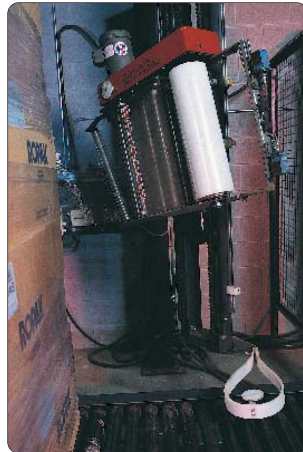
The Wulftec Tornado 200 installed at the Ropak plant in Oakville has several custom built-in features that allow it to optimize load stability and virtually dispense with the use of wooden pallets altogether.
