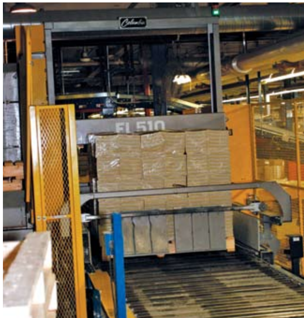
One of two Columbia Machine FL510 floor-level palletizers takes bundles of printed materials and neatly stacks them on a pallet.
